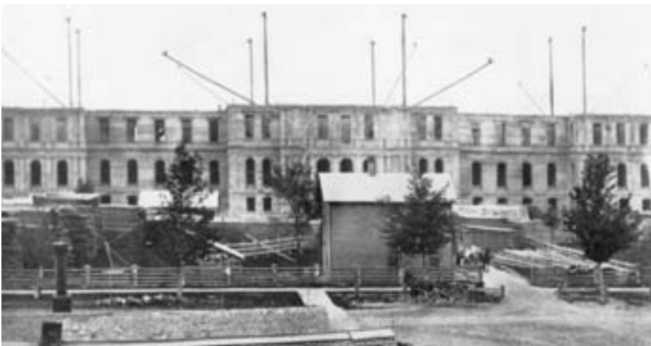
The Capitol under construction in 1875. Derricks rise above the walls, which have been completed to the second story.
